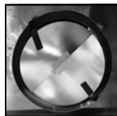
Black Tape on Damper
