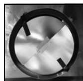
Black Tape on Damper
